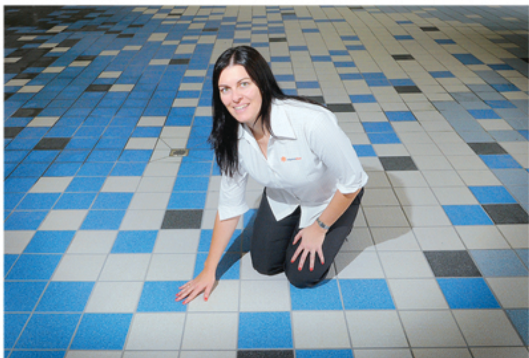
SAFER FOR PATROLS: Mildura Waves centre manager Michelle Lyons has a look at the new tiles in the pool.
